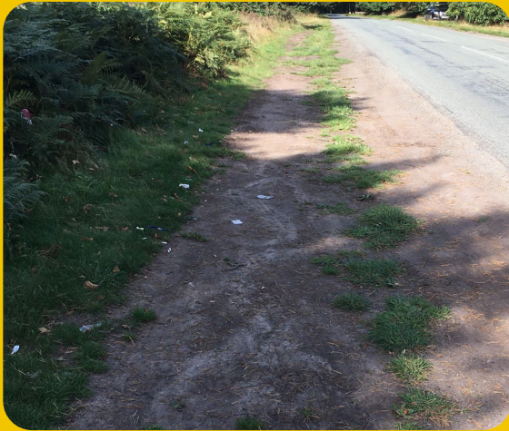
Damaged verge, Brindly Heath Road
