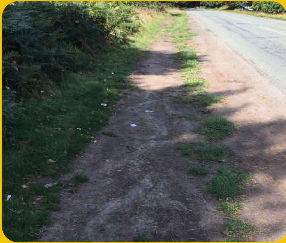
Damaged verge, Brindly Heath Road
